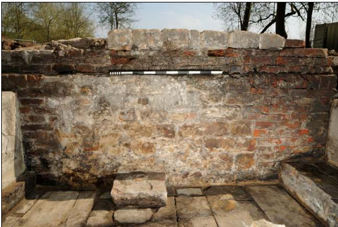
Plate 10: Area C detail of engine room north facing wall (045) and red brick rebuild (072) with (040) in the foreground. Photo Adam Stanford
